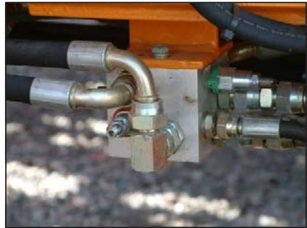
Fig. 5.06: Pro-Lift Tine Hydraulic Manifold
